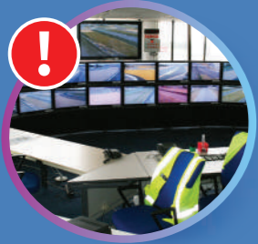
Neighbourhood central monitoring station
